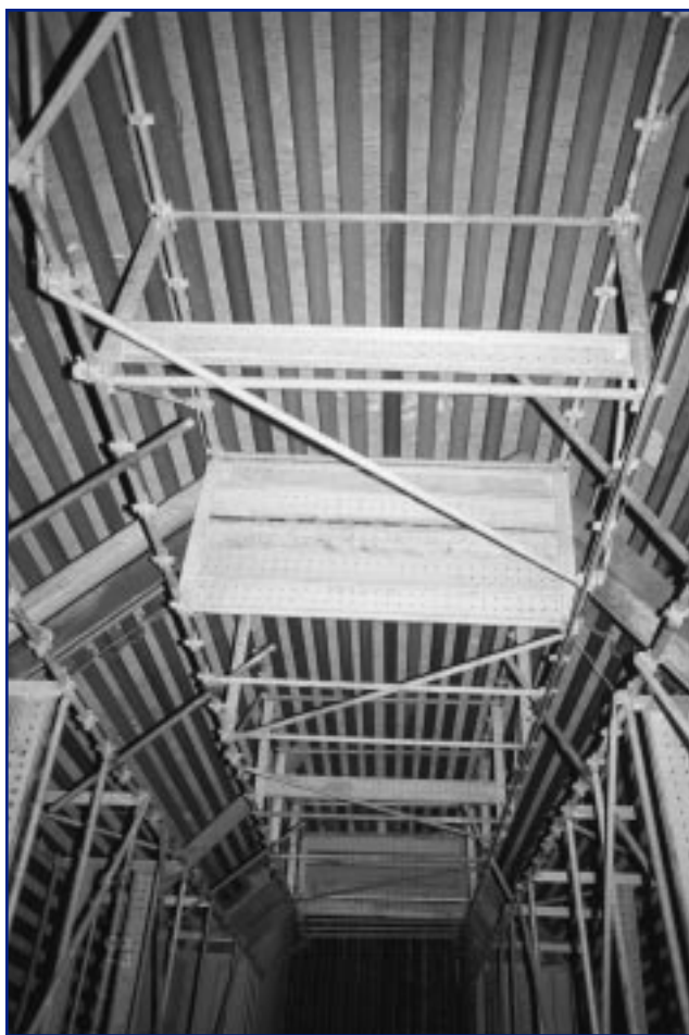
Photo 3 Vertical Cylindrical Heater
