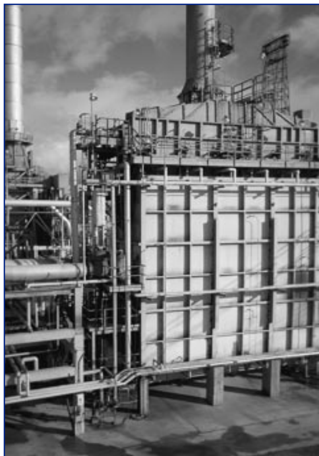
Photo 2 Outlet Tubes Exit Middle of Heater
