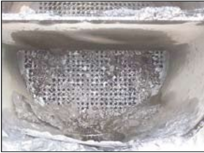
Figure 2 Fouled exchanger tubes — asphaltene precipitation
