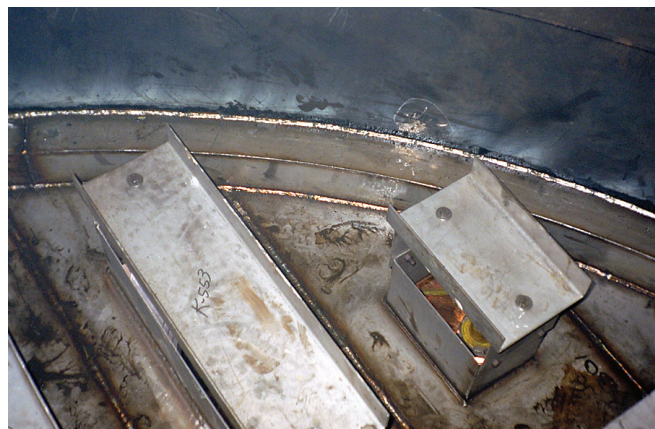
FIG. 11. Revamped depentanizer with view of the reboiler feed tray.
