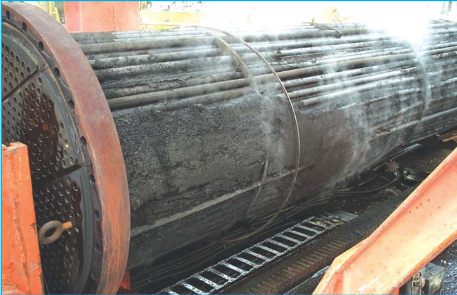
Photo 2. Debutanizer reboiler shell-side fouling
