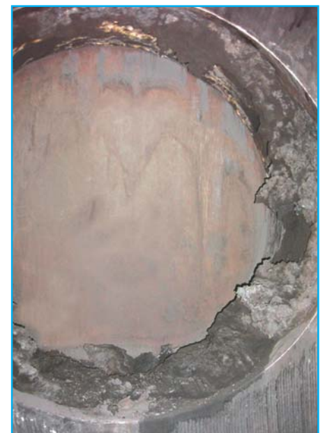
Photo 1. Reactor vapor transfer line coke
