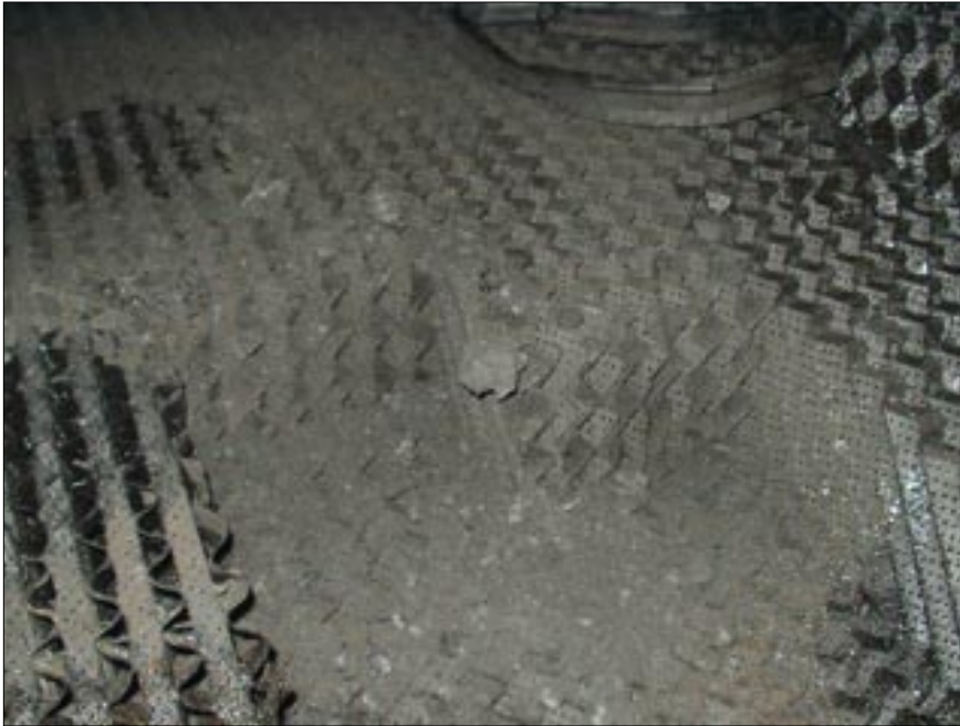
Figure 3 Severe wash zone coking
