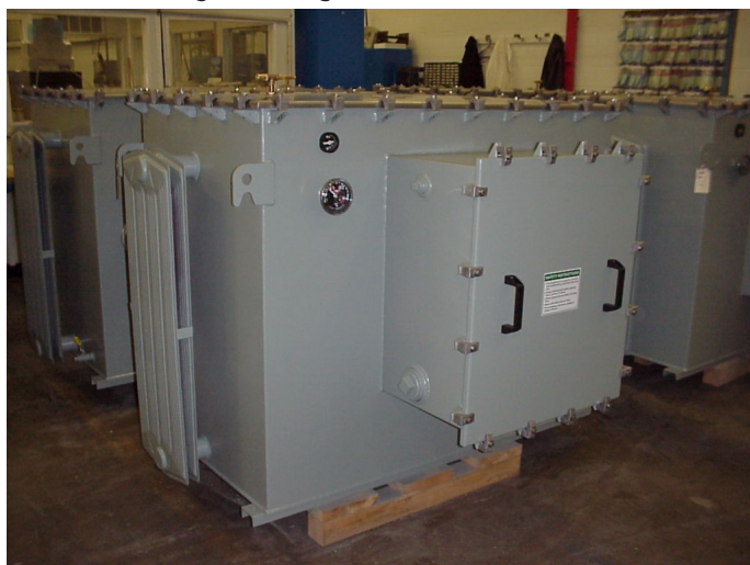
Figure 3 Large Power Transformer
