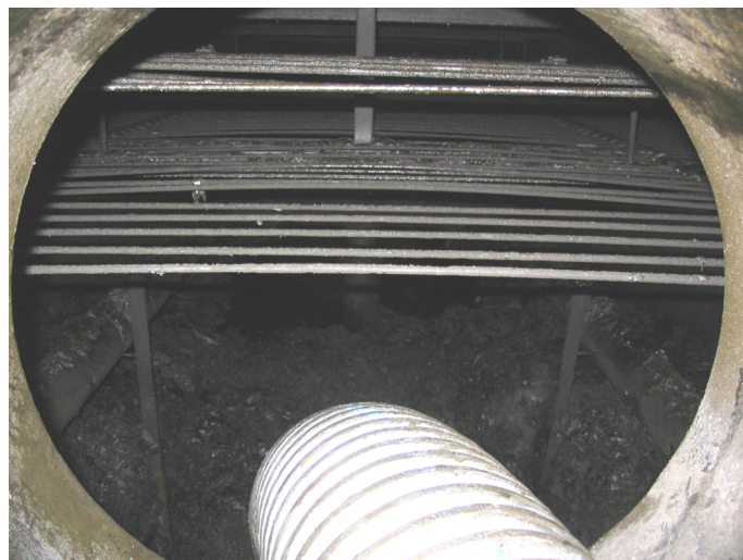
Figure 4 Large Accumulation of Sludge
