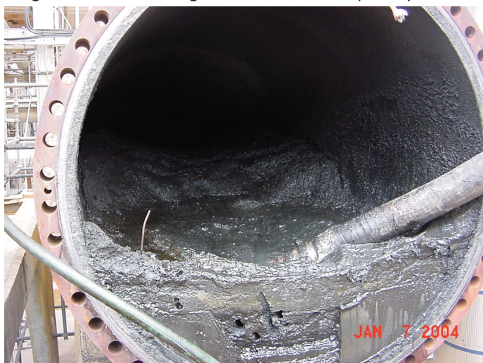
Figure 1 Severe Fouling in Crude Column Top Pumparound
