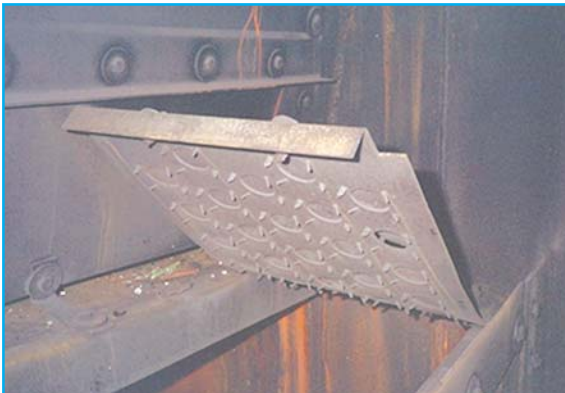
Photo 2. Damaged stripping section trays
