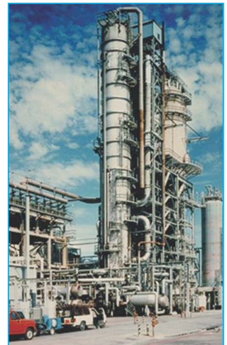
Photo 3. Packed FCC Column
