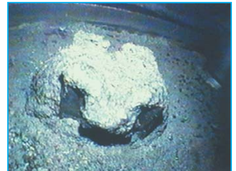
Photo 7. Collector Tray Coking
