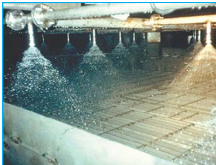
Photo 6. Spray Header Testing
