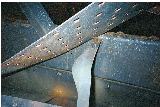
Fig. 11. Damaged stripping trays.
