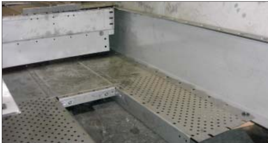
This efficient, low-fouling tray was used in the revamped stripping section (Fig. 10).
