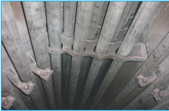
Photo 3. Shock Tubes (Bridgewall Temp.)
