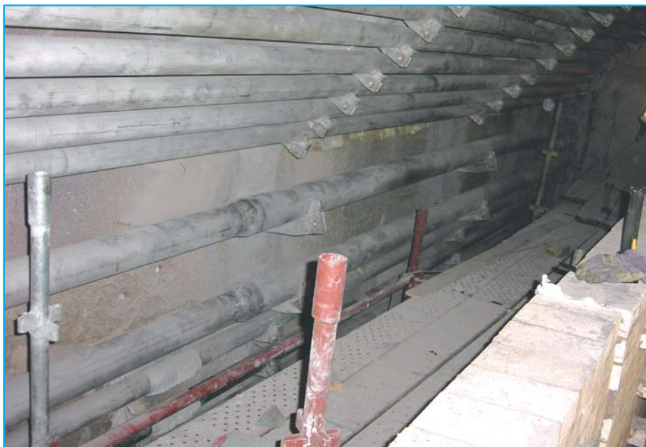
Photo 7. Heater Outlet Tubes
